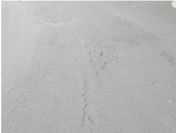
Broken Arrow St (PCI = 50, Poor)
