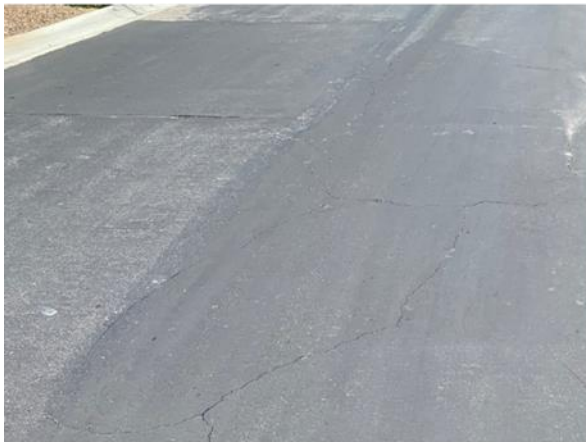
Oberon Rd (PCI = 74, Satisfactory)
